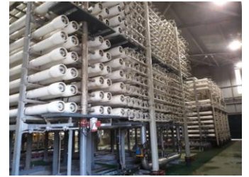
LARGE DESALINATION 60,000M3D
