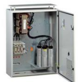
Power Factor Correction 20% energy
